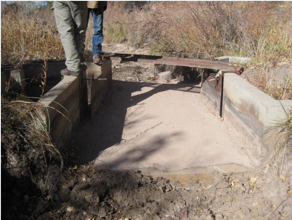
Photo 1: Typical division box used to divert water from the ditch.
