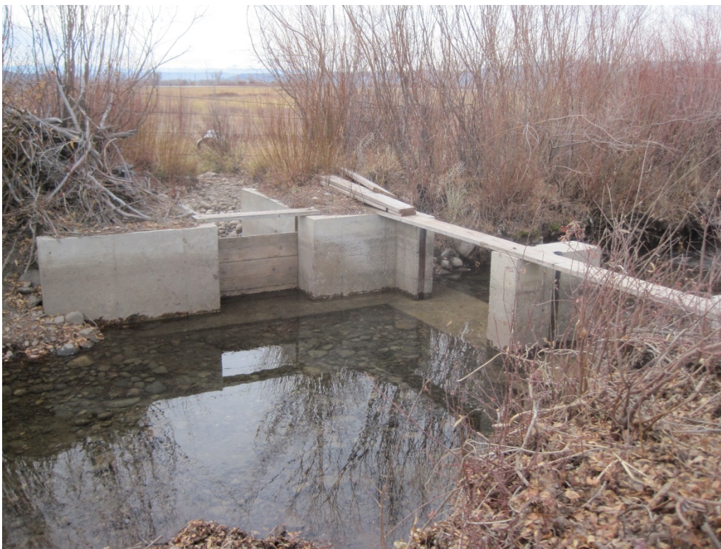
Photo 1: Typical irrigation diversion from the canal.
