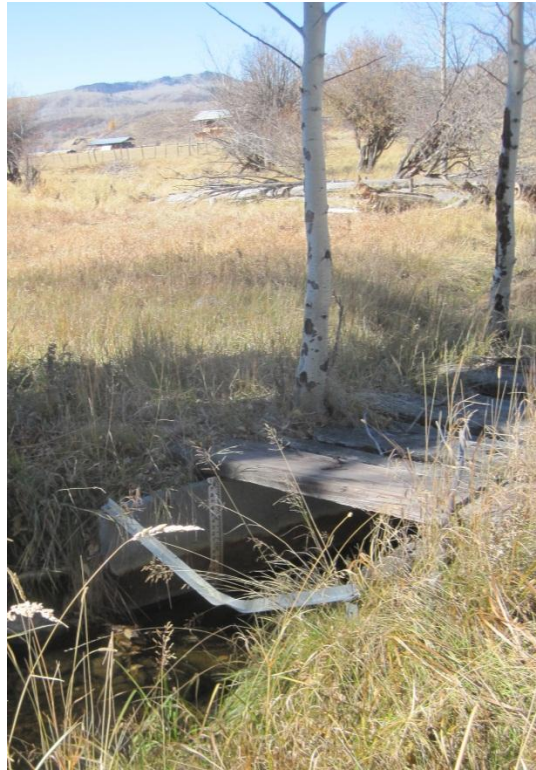
Photo 3: Ekhart Ditch Parshall flume.
