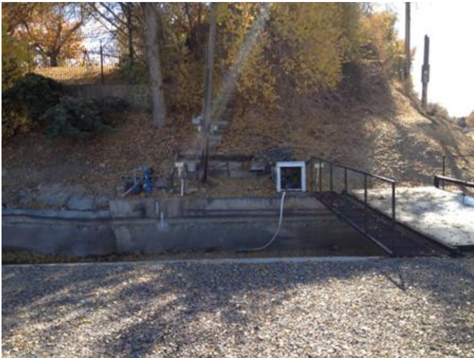
Photo 1 Typical Residential Irrigation Pumping Station from the Grand Valley Canal.
